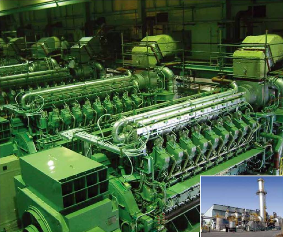
Backbone power of Higashida Area using natural gas
